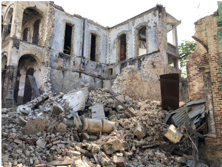
Building damaged by the earthquake in Haiti, August 2021.
